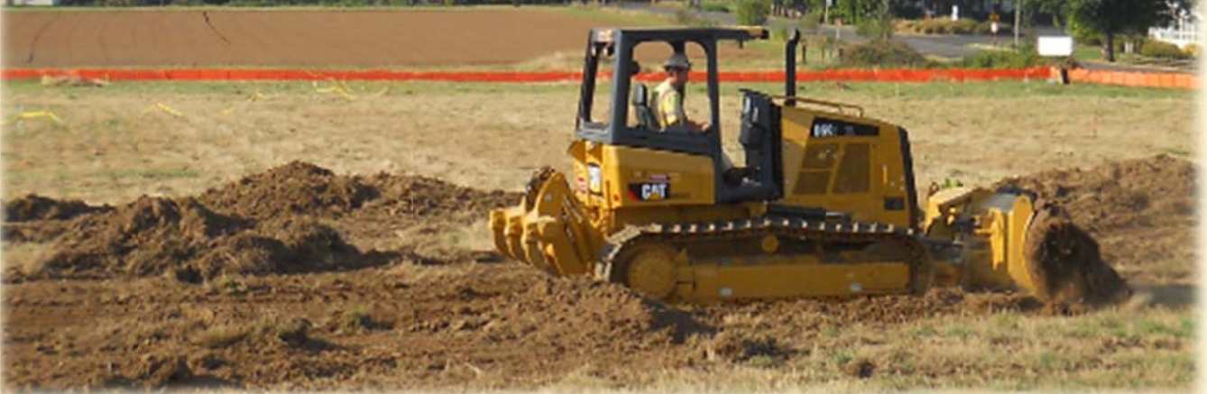
Benny operates the dozer to strip off the top layer of grass
