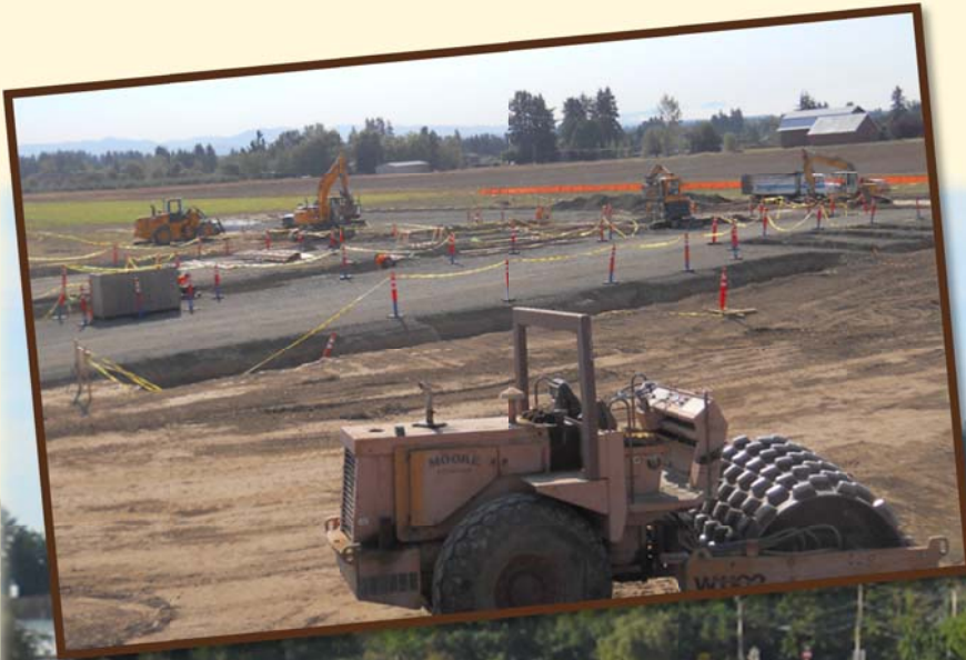
Equipment hard at work to get the site ready for a new Fire Station
